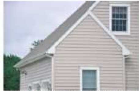
Pork Chop Cornice Return – Unacceptable
