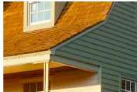
Colonial Cornice Return – Acceptable
