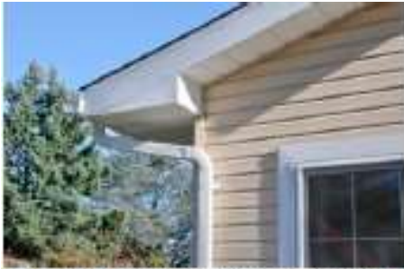
Pork Chop Cornice Return – Unacceptable
