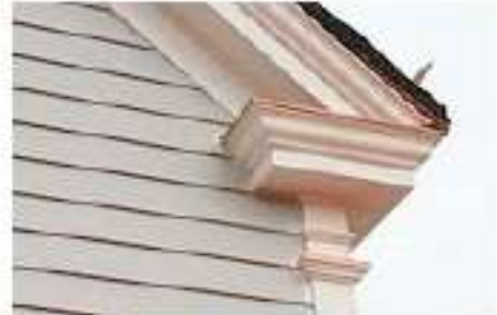
Greek Cornice Return – Acceptable
